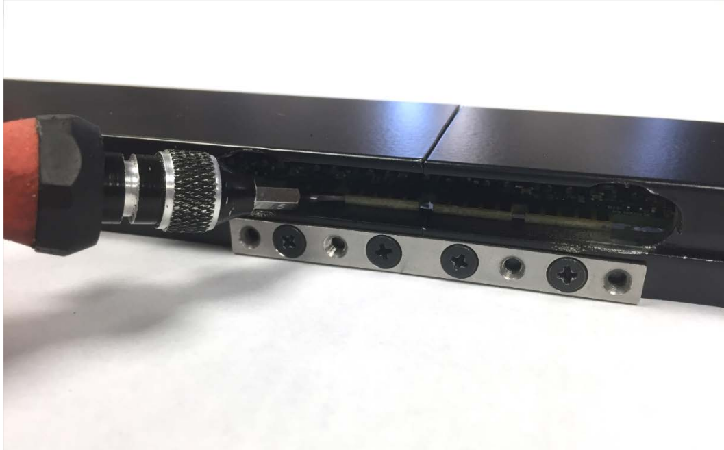
Figure 21: Using a Screwdriver to Nudge Circuit Boards into Alignment
